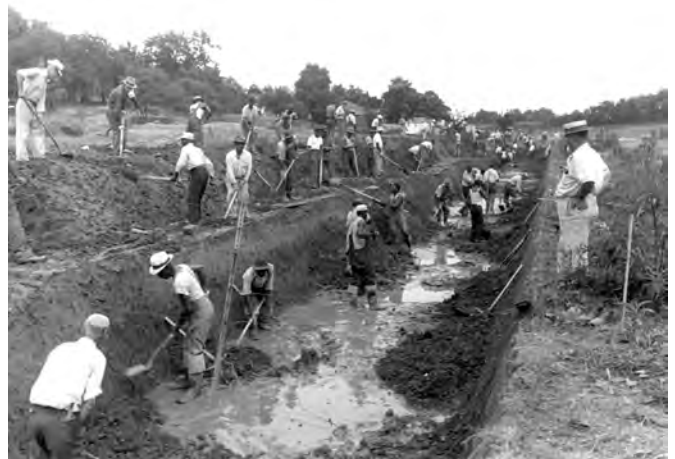
In 1940, the federal Works Progress Administration paid day laborers to dig the trench in which the Beals Branch sewer would be constructed.
